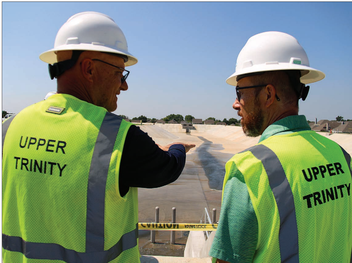
Construction Project Manager Chris Jones, left, and Jason Pierce, manager of governmental affairs and communications for Upper Trinity Regional Water District, look over the diurnal pond as it fills for the first time on July 11 at the Tom Harpool Water Treatment Plant in Providence Village.
