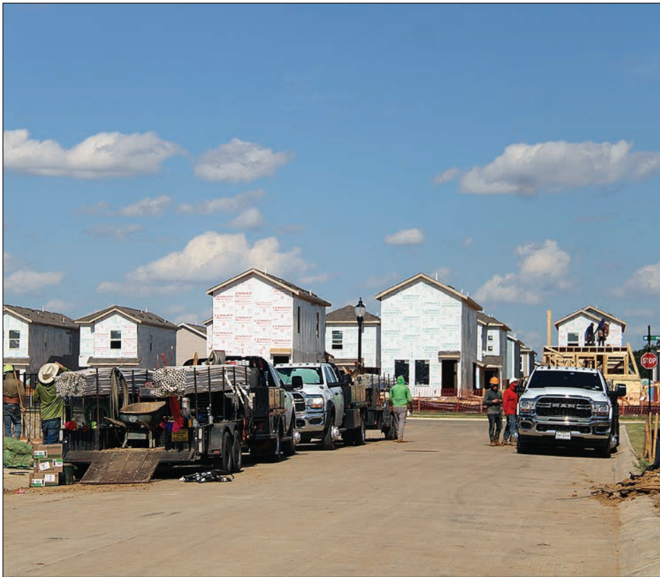
Crews work on the construction of several types of homes in the Lennar-developed Foree Ranch in Providence Village.
