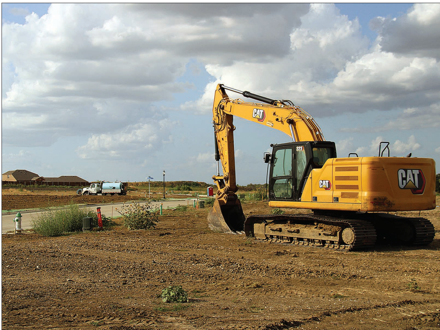
An excavator sits waiting for its crew in the Creekview Meadows development, south of neighboring Moberly Farms. Both developments will have thousands of homes within them at buildout.
