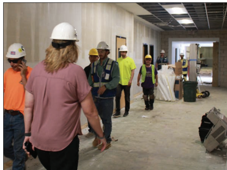
Aubrey ISD Superintendent Dr. Shannon Saylor leads the way through the high school’s recent renovations. The changes will improve functionality and double the campus’ capacity.
